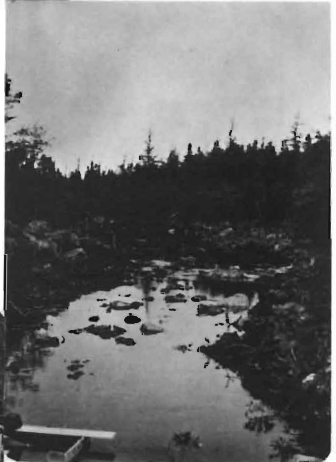
Photo No. 9 - River run-around with the foundation of the first outside raceway.
