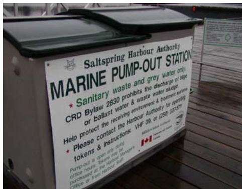
Saltspring Harbour Authority Pumpout Facility
