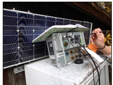
Image 2. Real time water temperature logger installation on Stuart River.
