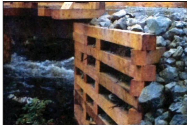
Figure 3.30 Infill materials for timber cribs should be blocky, angular and free of fines or sediment.
