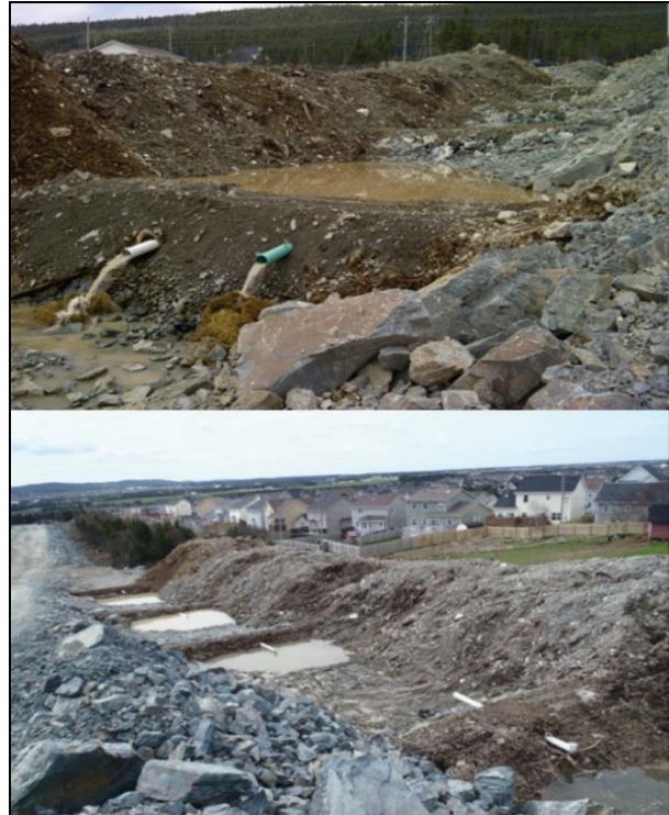
Figure 3.8 View of a series of settling ponds (top and bottom images).
