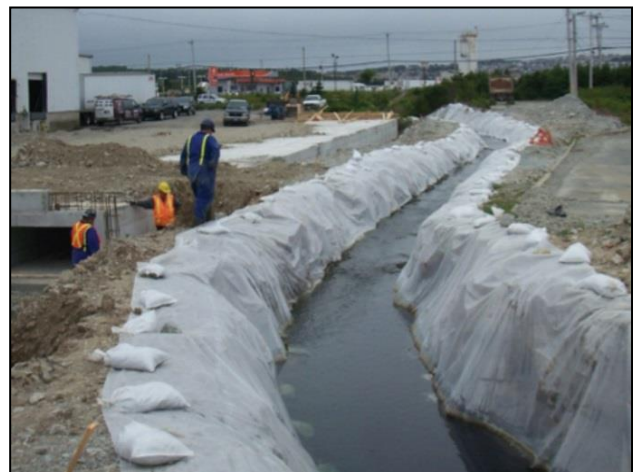
Figure 3.40 Temporary diversion channels should be lined with plastic that is weighted down with stone.
