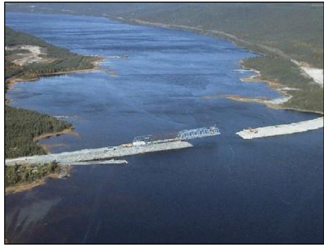
Figure 3.32 Aerial view of Alexis River bridge and causeway constructed along the Trans-Labrador Highway. Photo credit: G. Jin et al. 2003
