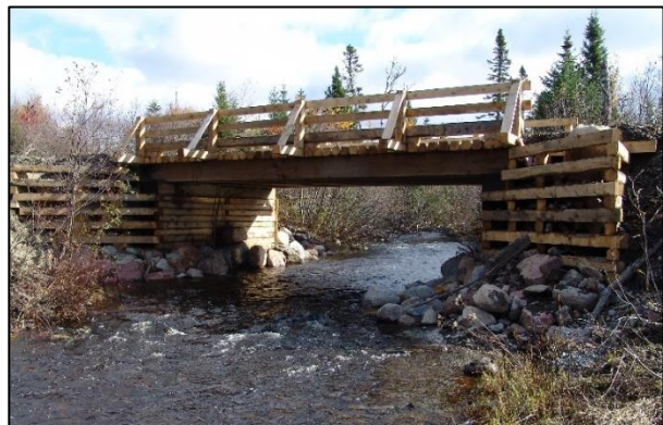
Figure 3.31 Untreated or pressure treated wood should be used for timber crib construction.
