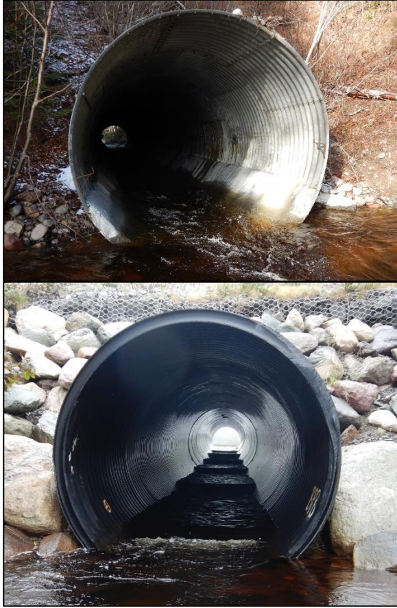
Figure 3.28 Examples of repaired culverts (top image shows concrete reinforcement and bottom image shows HDPE liner).
