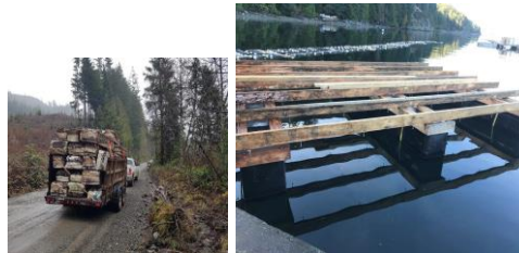
Collection of replaced styrofoam rafts going to disposal and installed durable alternatives.
