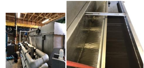
Installation of an advanced oxidation process to remove color and solids from wastewater and the clear effluent discharge.
