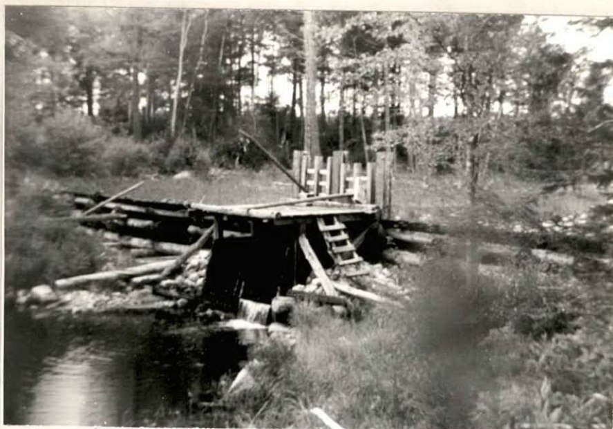
Photo 15. Former driving dam at Croker Lake in the headwaters of the main river.
