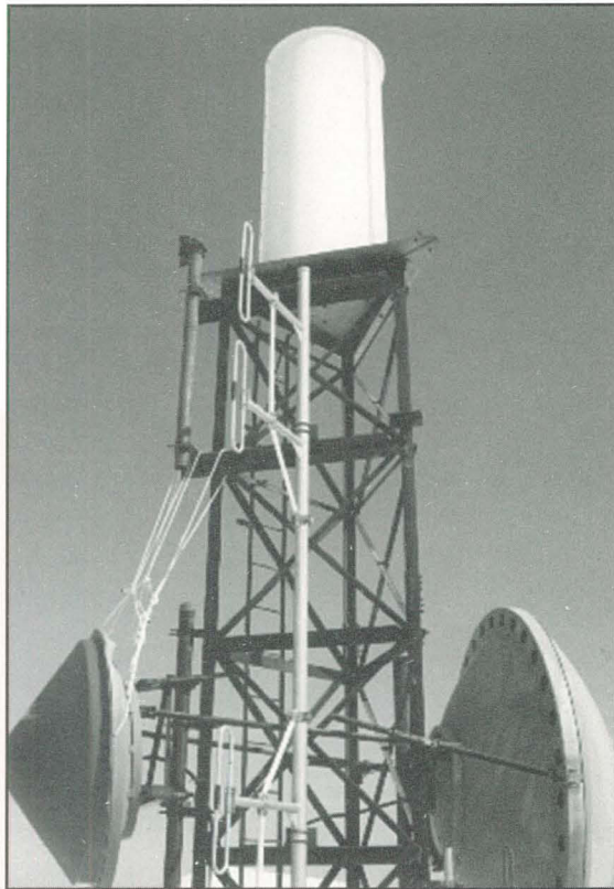
The results of eight months of winter weather so severe that seven of eight dipole antennas were lost and the last one was hanging by a piece of rope and some cable. All were replaced.
