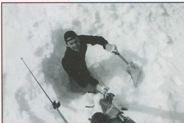
Lesson one: before you can repair a cable, you must first find it! Ernie Quiring shovels and sweeps to find the object of his repair at Van Isle Inlet, April 10, 2000.
