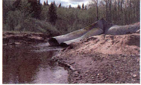
Washed out culverts on a forestry road crossing of Broad Creek in Alberta.
