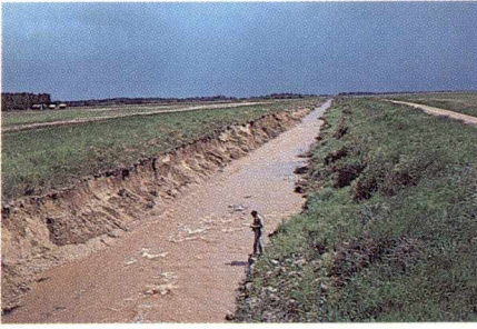
This gun-barrel-straight drainage ditch, built to get water off farmland faster, encourages erosion and eliminates the diversity of habitat necessary to support many fish species.
