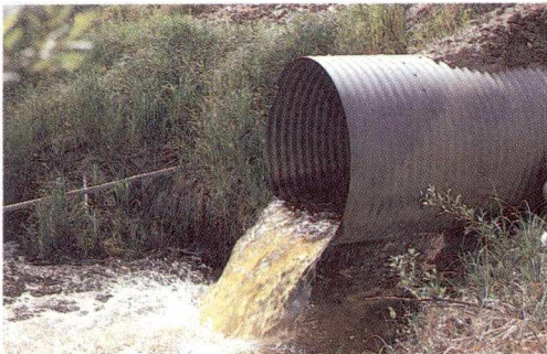
This culvert installed at Trapper Cabin Creek in Saskatchewan prevents fish passage by creating a waterfall. Culverts with high velocity flows also present a barrier to fish.
