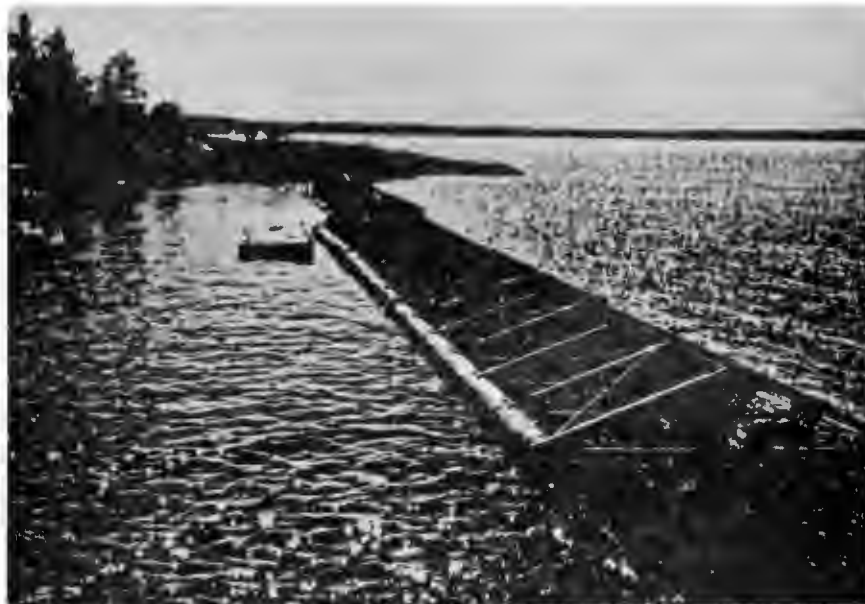
A. Breakwater at Lund, B.C., with centreboard support frames above water level
