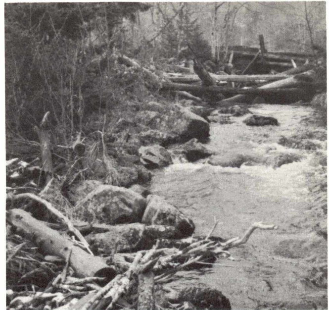
A site at the outlet of Grand Lake, Musquodoboit River, Nova Scotia, where stream clearance work is proposed.
