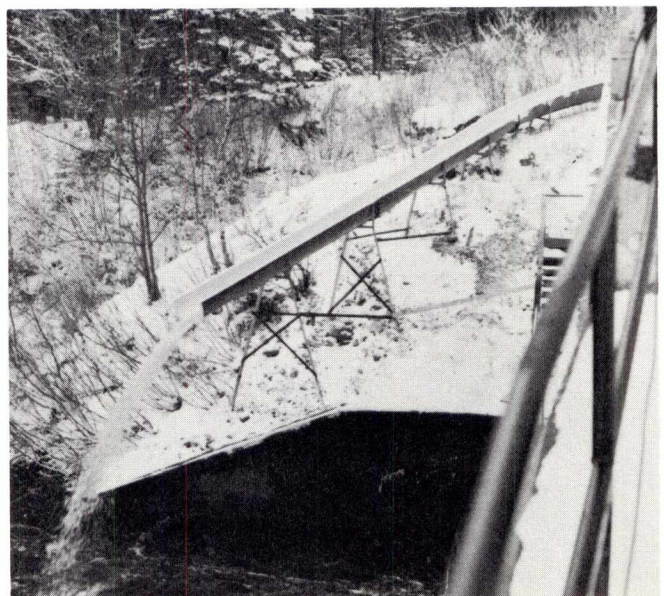
Fiberglass flume, carrying smolts from deflector screen, around turbines and to the tailrace.
