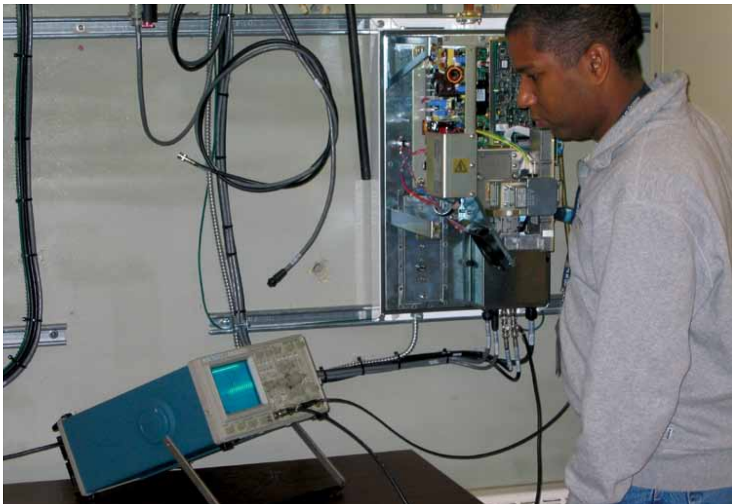
Senior Technologist, Milo Ewing, performs annual maintenance on the harbour surveillance radar system.
