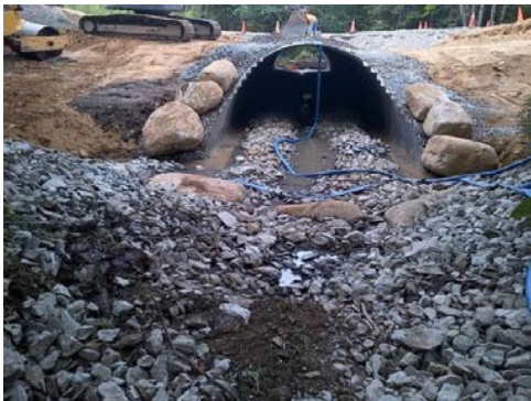
Figure 4. Example of a poorly installed open-bottom structure.
