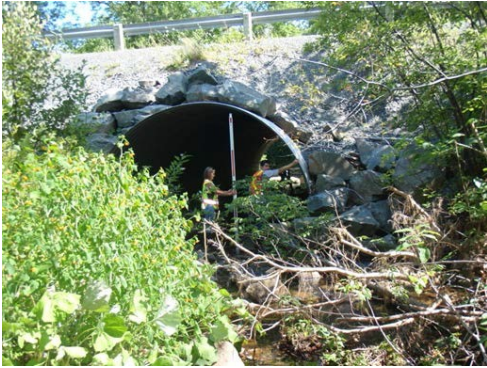
Figure 22. Example of a culvert in need of remediation
