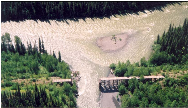
Figure 119. Skeena–Duti confluence. Photo shows washed out BC Railway bridge
