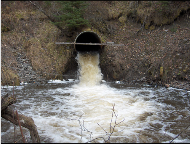
Figure 122. Station Creek culvert with 1.5 m outfall drop. This culvert passing under Highway 16 does not allow fish passage.
