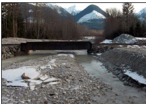
Figure 34. Shames River sediment accumulated under CN Rail bridge.
