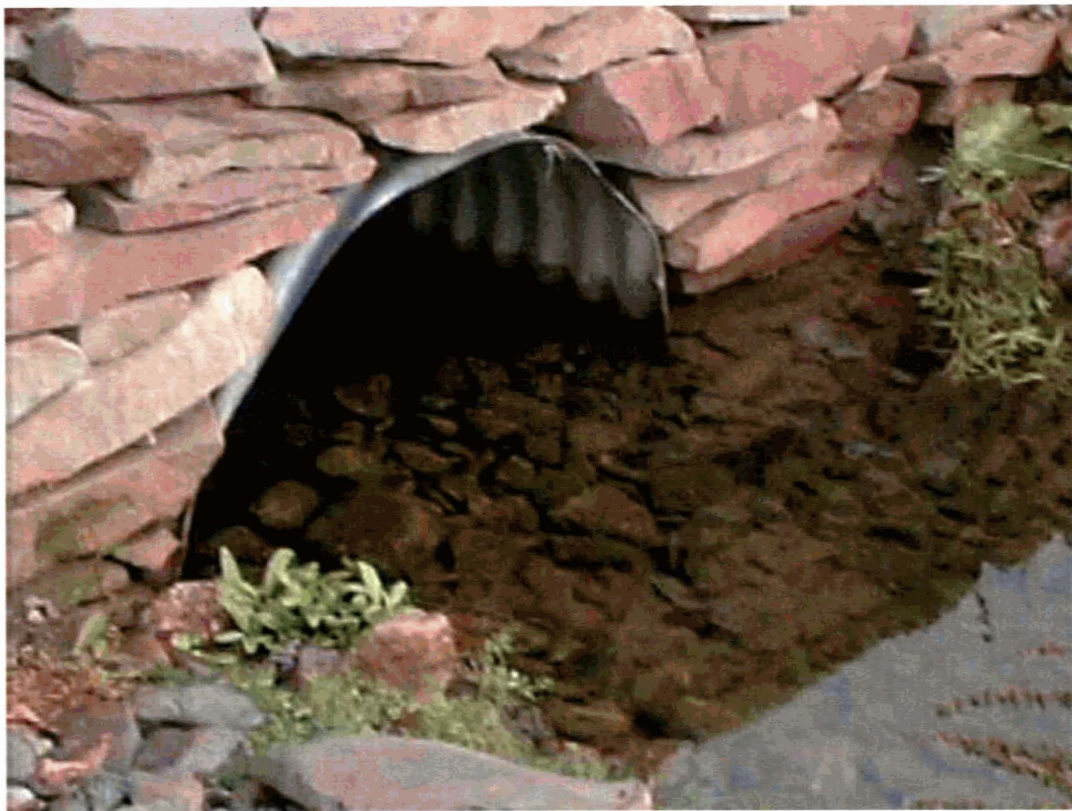
Figure 16: Culvert being filled by bed load material from above culvert site.
