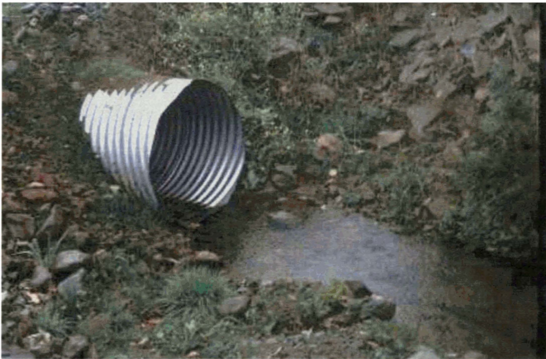
Figure 13: Riparian vegetation not re-established as required.
