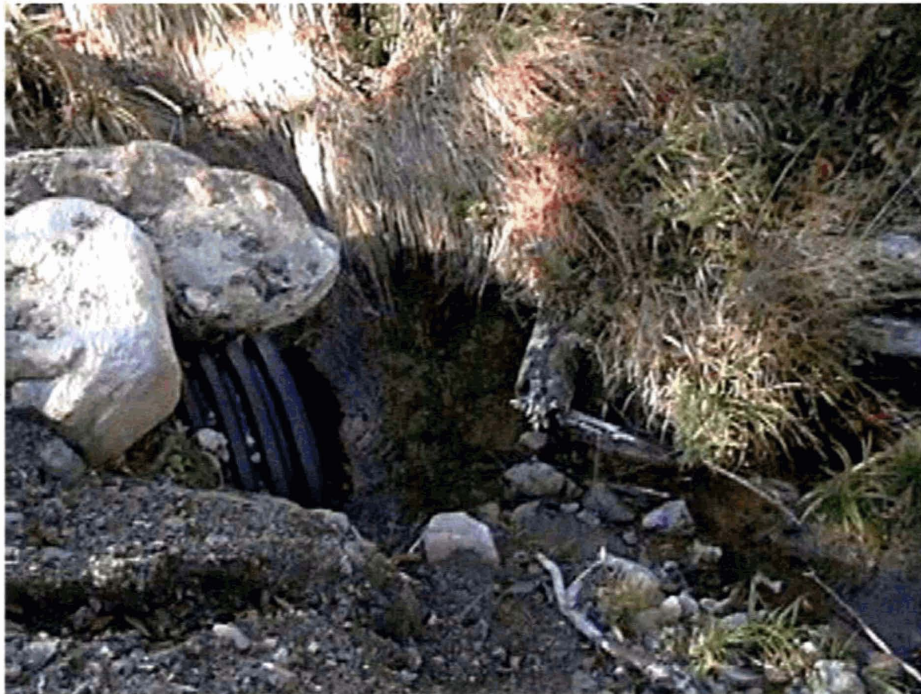
Figure 9: Culvert end not properly protected.
