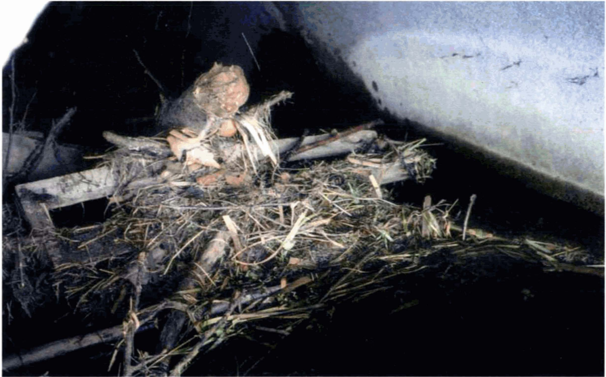
Figure 8: Debris blockage obstructing fish passage.
