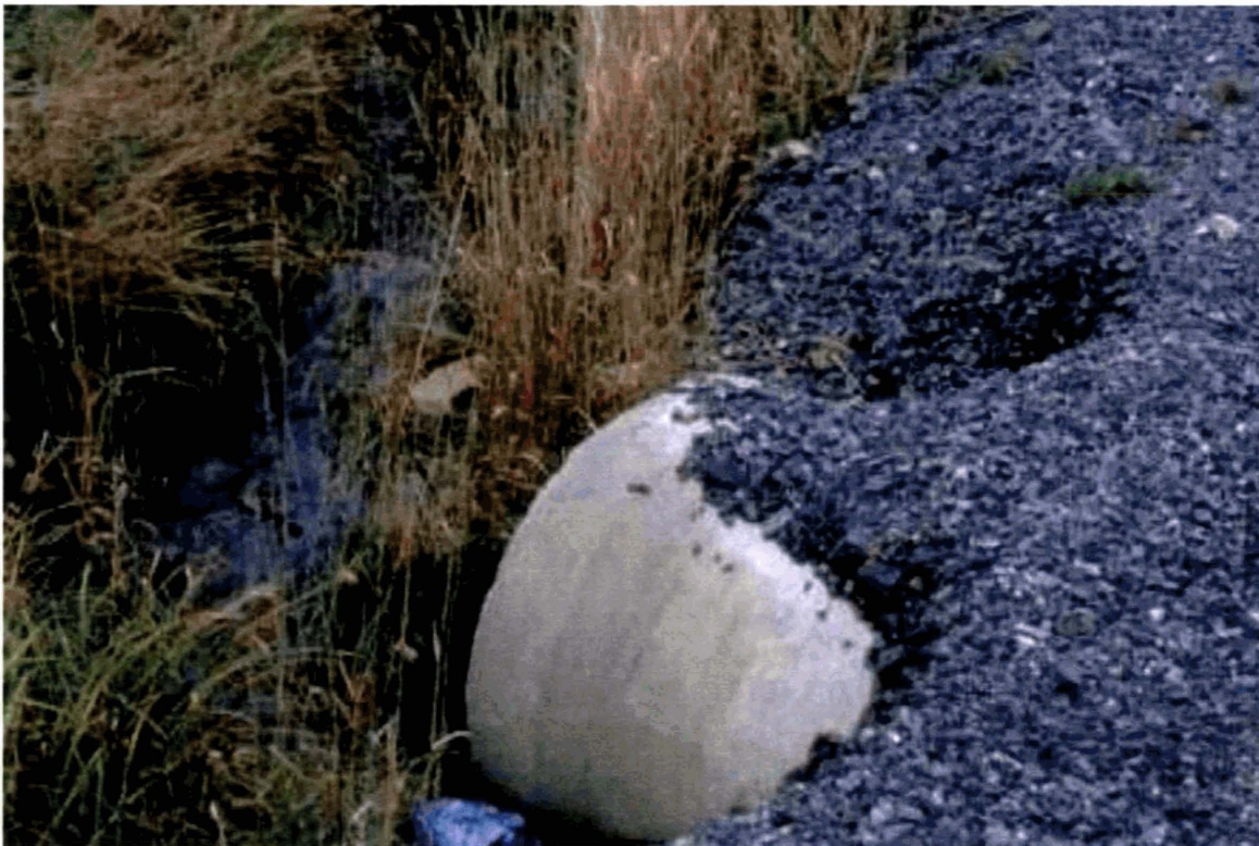
Figure 14: Inappropriately installed culvert resulting in road failure.
