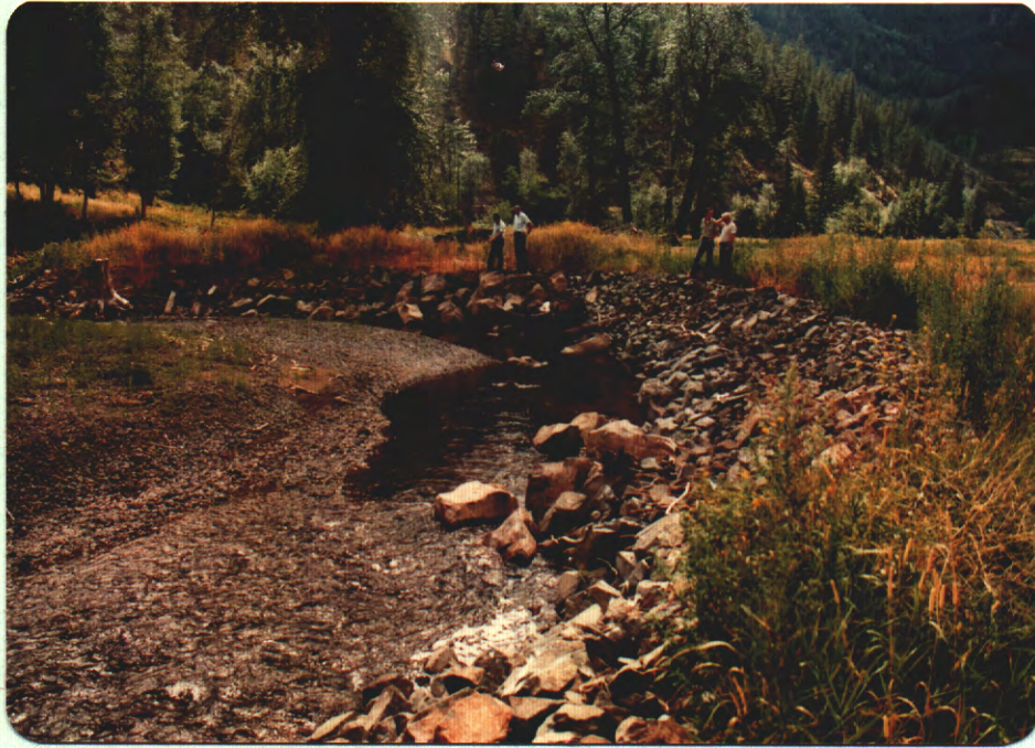
PHOTO 9. Rip rap placement in the Deadman River where bank protection and mitigation works have occurred to reduce erosion rates (Photo by G. Kosakoski).
