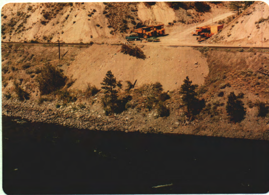
PHOTO 8. Widening the railway track with material sidcasted in the Thompson River upstream of the Nicola River confluence (Photo by G. Kosakoski).
