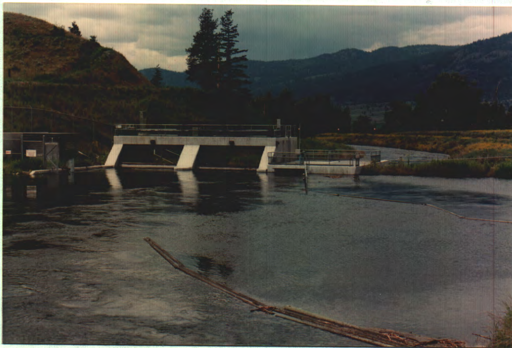
PHOTO 4. Downstream view of the Nicola Lake Dam, June 1990. (Photo by J. Patterson).
