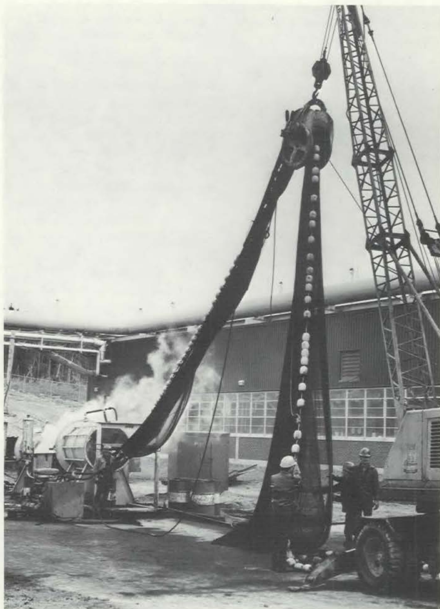
The steam laundry specially constructed to clean oil from seine nets, shown in action at Point Tupper, N.S.
