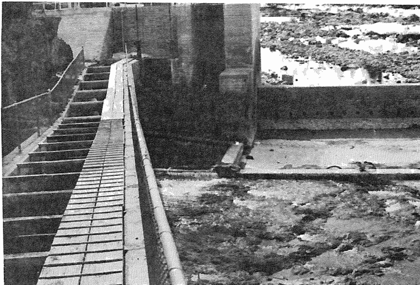
Plate 91. Entrance to the fishway at low water (note barrier dam to right).
