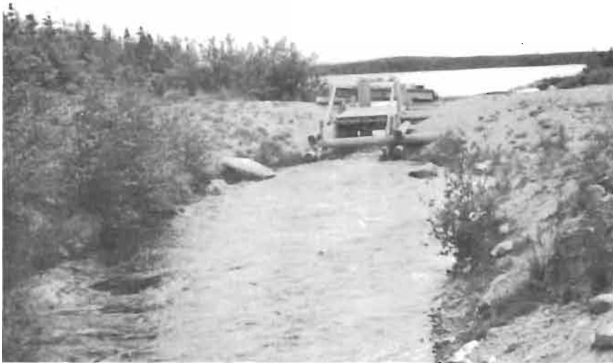
Figure 3. Controlled-flow spillgate and diversion channel at the outlet of Paddys Pond.
