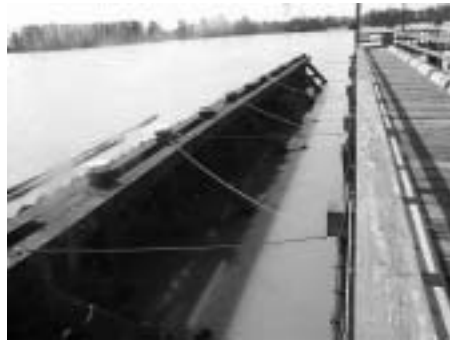
A debris shear at Mission, British Columbia, protects the wharf from floating debris. Note the concrete parking barriers and cabling on the wharf itself.
