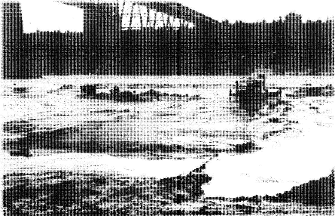
Figure 32. Bridge foundation excavation flooded by the increase in water level as the freeze-up pack progressed upstream past the site
