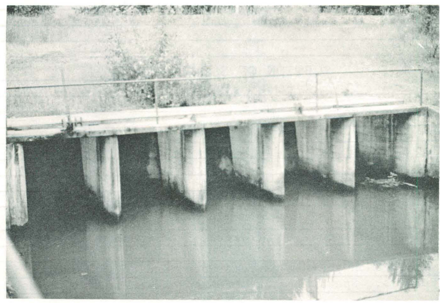
Upstream side of pump house facility on Chilliwack Creek.
