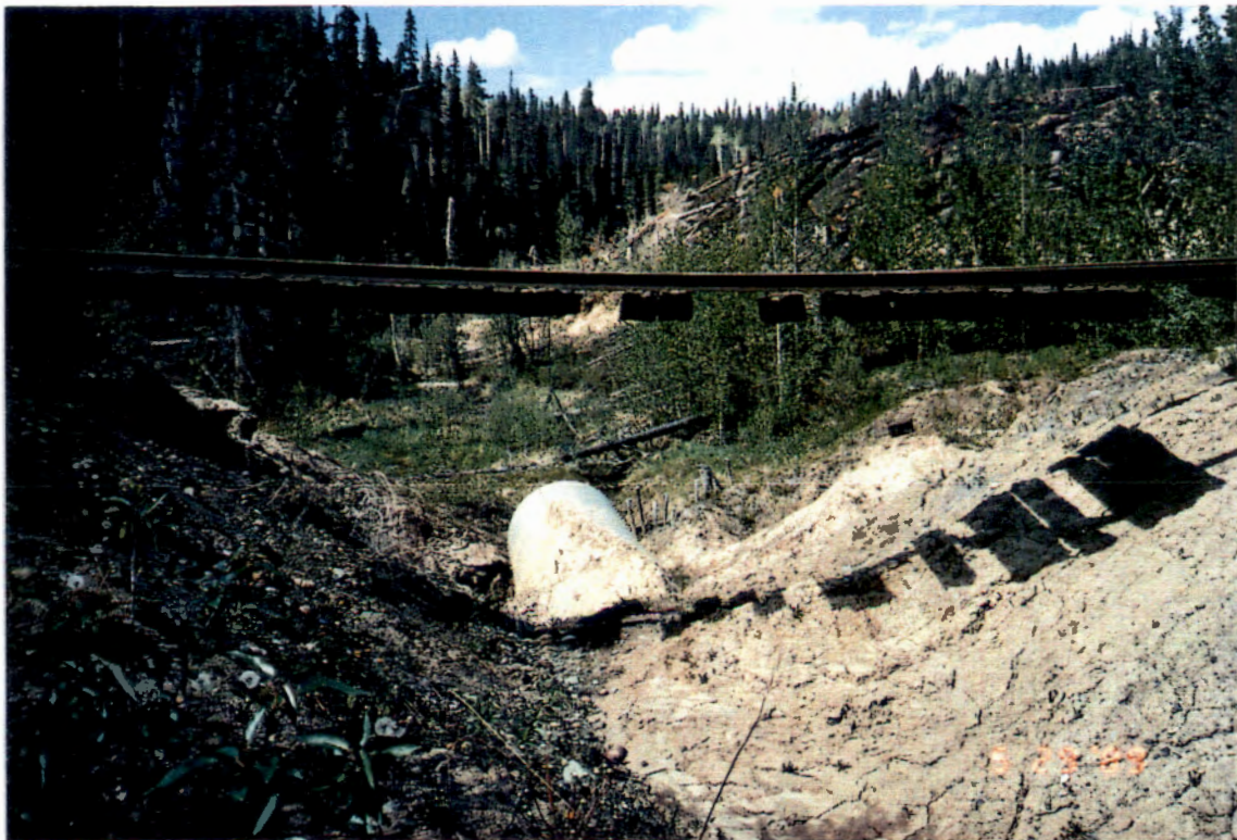
Figure 4.15 British Columbia Railway culvert washout on an unstable valley wall. Photo courtesy of B. MacDonald.
