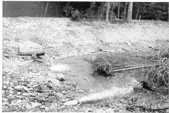
photo 1- Channel's Low and High Level Intakes
