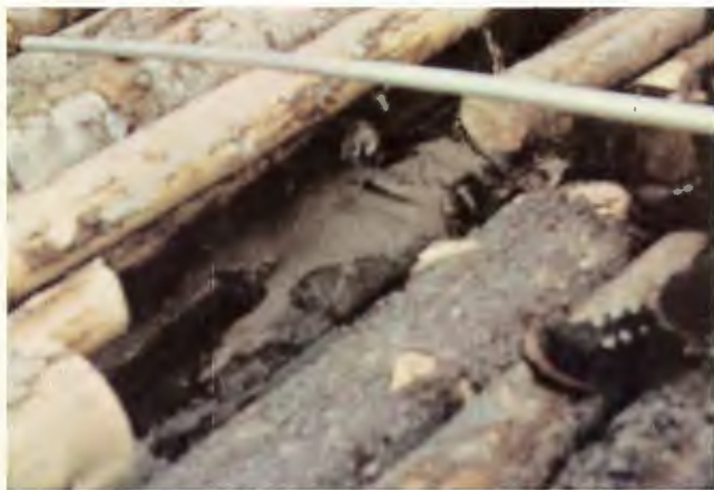
FIGURE 13—Silt deposited in a log jam in Area IX resulting from bottom and bank erosion in the vicinity.
