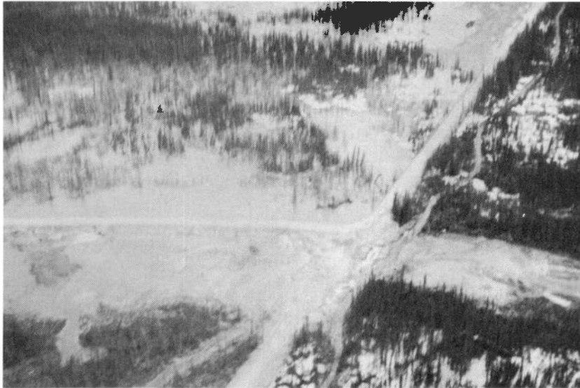
Figure 4. Accumulation of mill effluent at the angle between the two dykes, Pine Point, N.W.T., 1971. Two of the four decant culverts are visible. Stream flowing parallel to north-south dyke is pit water flow.
