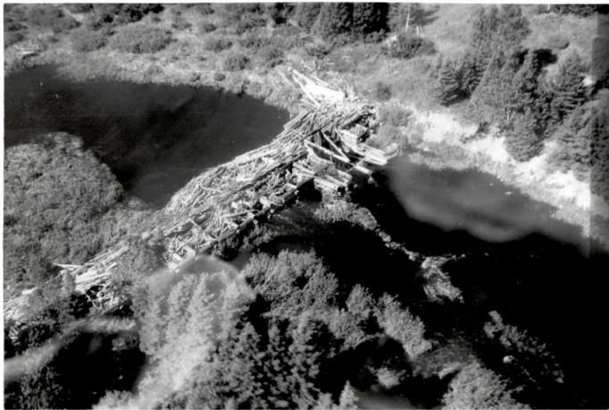
Figure 31: Deteriorated Dam - Tom Joe Brook.
