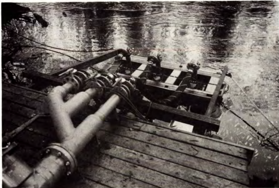
Fig. 8. Mathers surface water intake float with three electric submersible pumps, October 1981.
