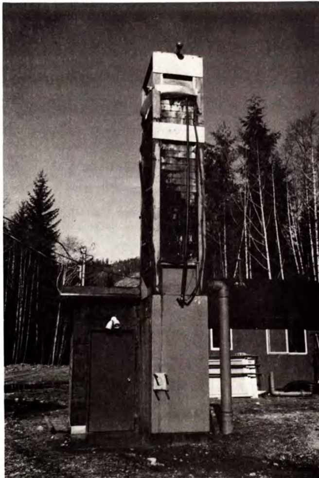
Fig. 10. Aeration tower with pumphouse (hatchery building is seen in the background), Mathers Creek pilot hatchery, October 1981.
