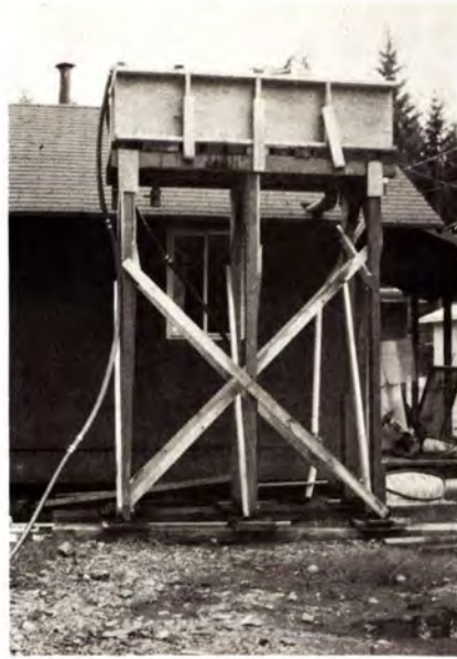
Fig. 9. Header tank used for settling of sediment in Mathers surface water supply, September 1982.
