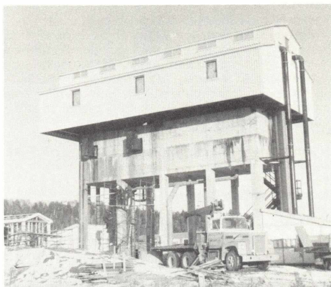
Newly modified aeration tower at Mactaquac Hatchery.
