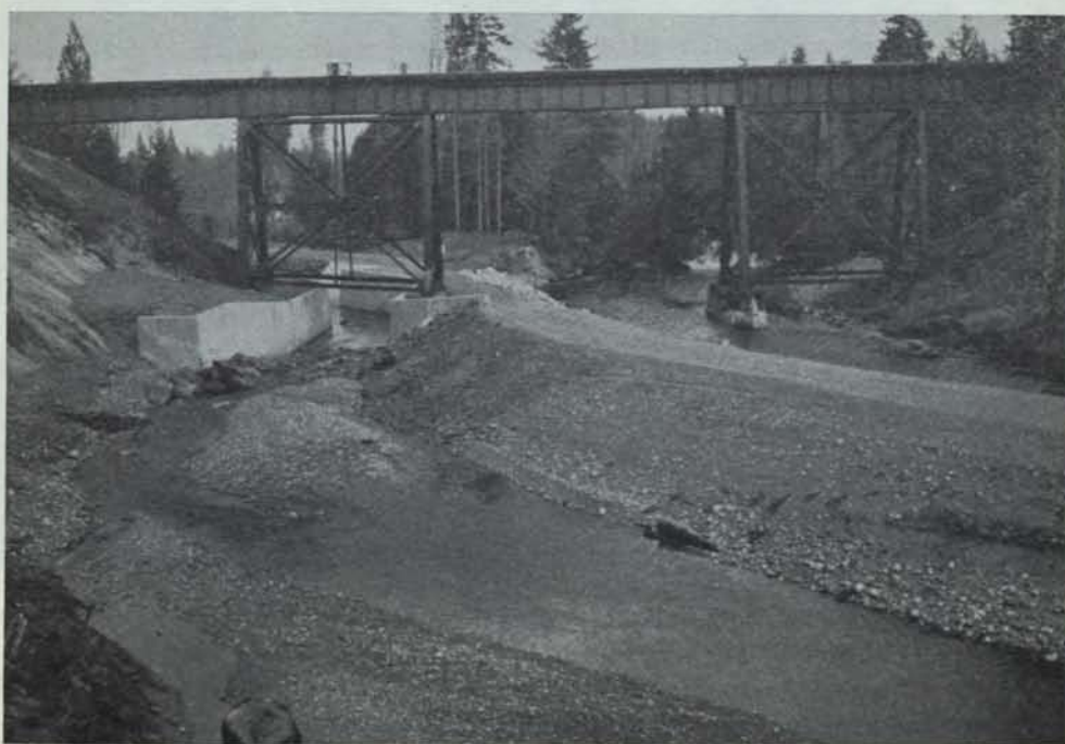
Concrete flume for Hunt's Creek flood channel under railroad bridge. Big Qualicum River at right.
