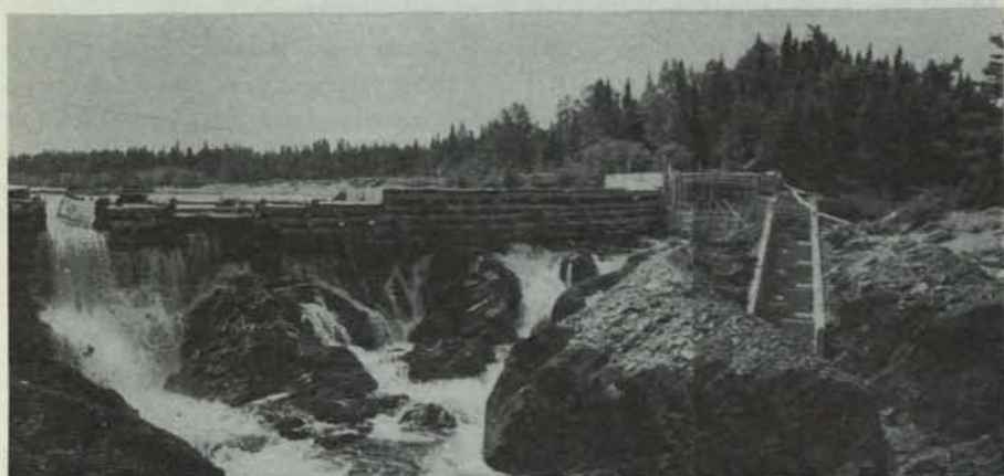
Nearly-constructed fishway on Great Rattling Brook, a major tributary of the Exploits River in Newfoundland. This fishway was built to allow the relocation of an entire run of Atlantic salmon, transferred from its original stream, Rattling Brook, to the headquarters of Great Rattling Brook by means of specially designed tanks carried on trucks. The installation will allow the progeny of the relocated salmon to reach the new spawning grounds. The transfer was made because hydro development on Rattling Brook threatened the continued existence of the run.
