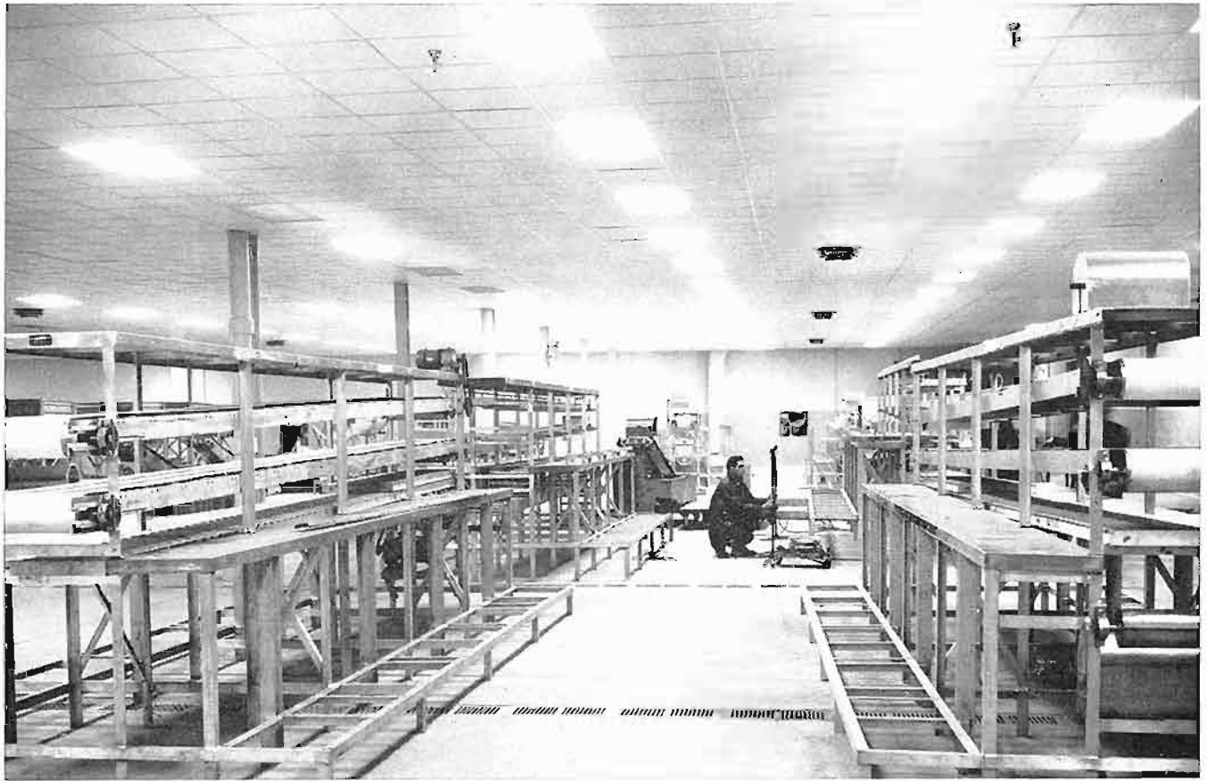
This photograph of two of the processing lines at Lunenburg Sea Products' new plant was taken during installation. Aluminum, stainless steel and plastics have been used exclusively to prevent corrosion.
