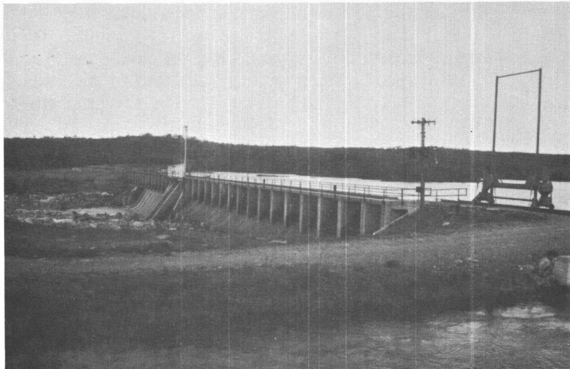
Fig. 3. Ruth Falls Dam, East River, Sheet Harbour, built in 1923 and rebuilt in 1964-65.
