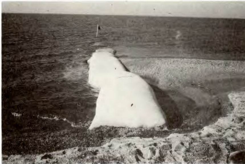
Plate 1. FABRICAST MOLDED BLOCK GROUYNE AS IT APPEARED FIFTEEN DAYS AFTER CONSTRUCTION (PHOTOGRAPHED AUGUST 3, 1978)
