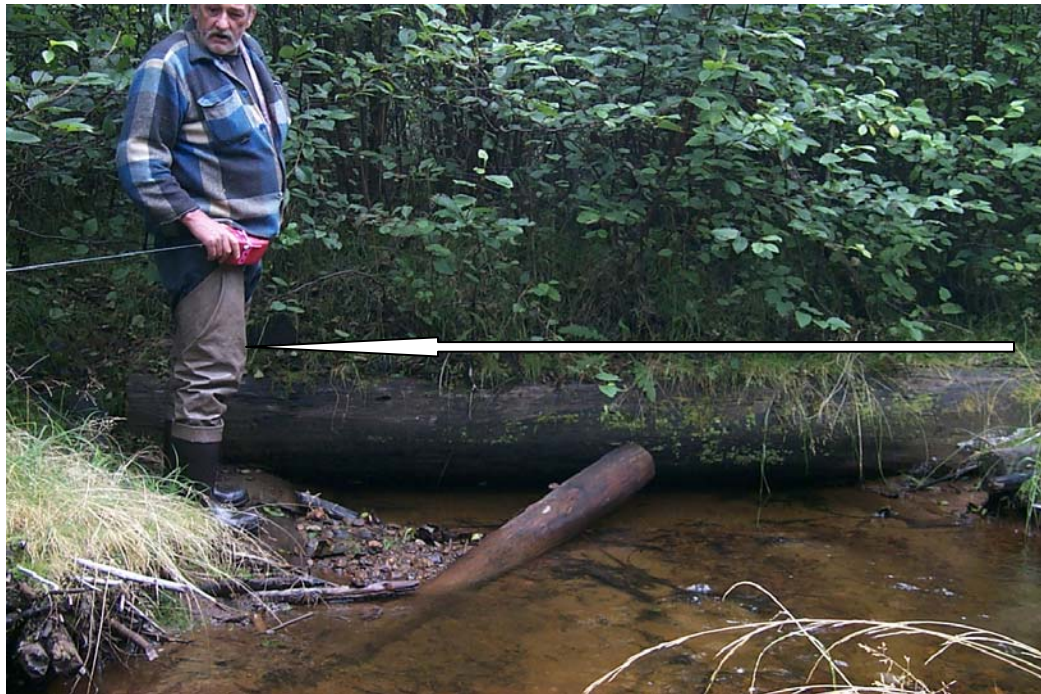
Photo 10: 0+192 m. Looking UP at collapsed wooden culvert (arrow runs along culvert).
