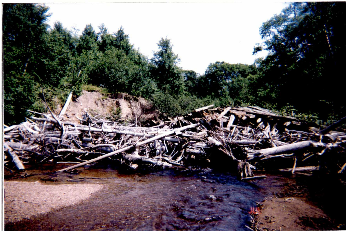
Collapsed Bridge on Clarkes Brook
