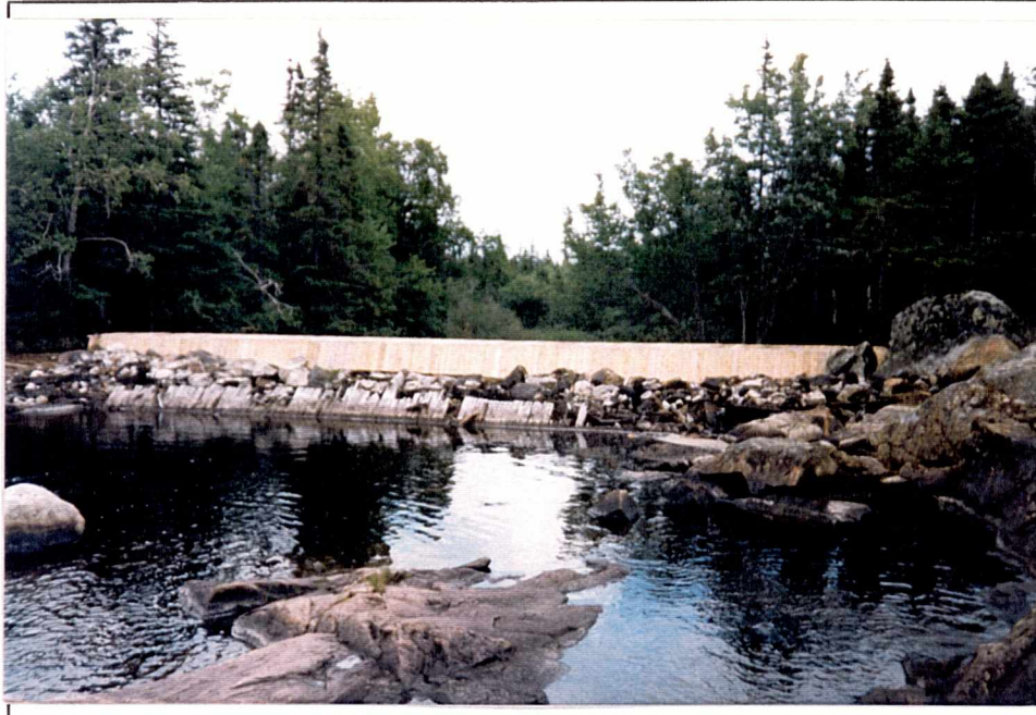
The old dam was used as a cofferdam as new dam was constructed.
