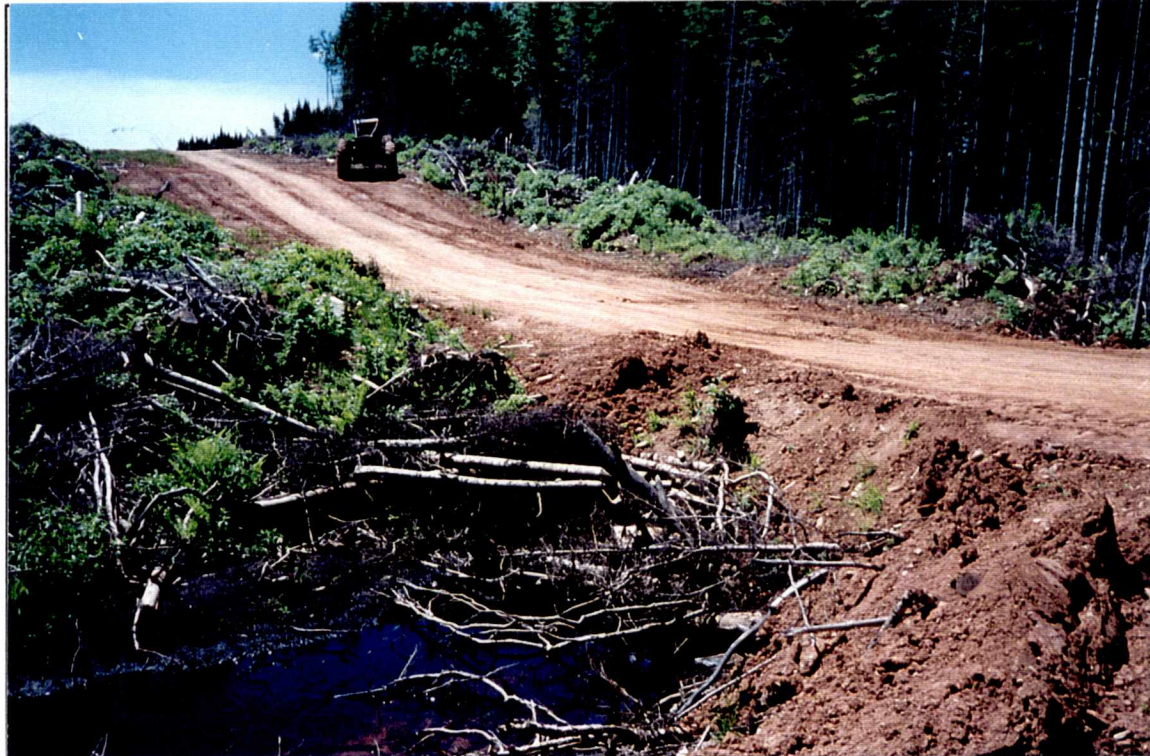
Improper forest road construction along the Humber River
