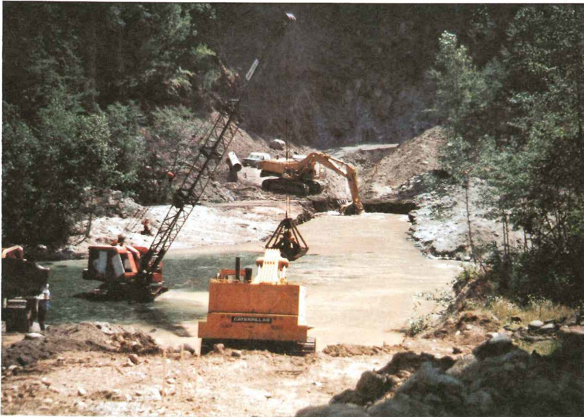
Heavy equipment used to excavate the stream crossing for a gas pipeline stains the Coquihalla River with brown silt. Photo: Ron Ptolemy
