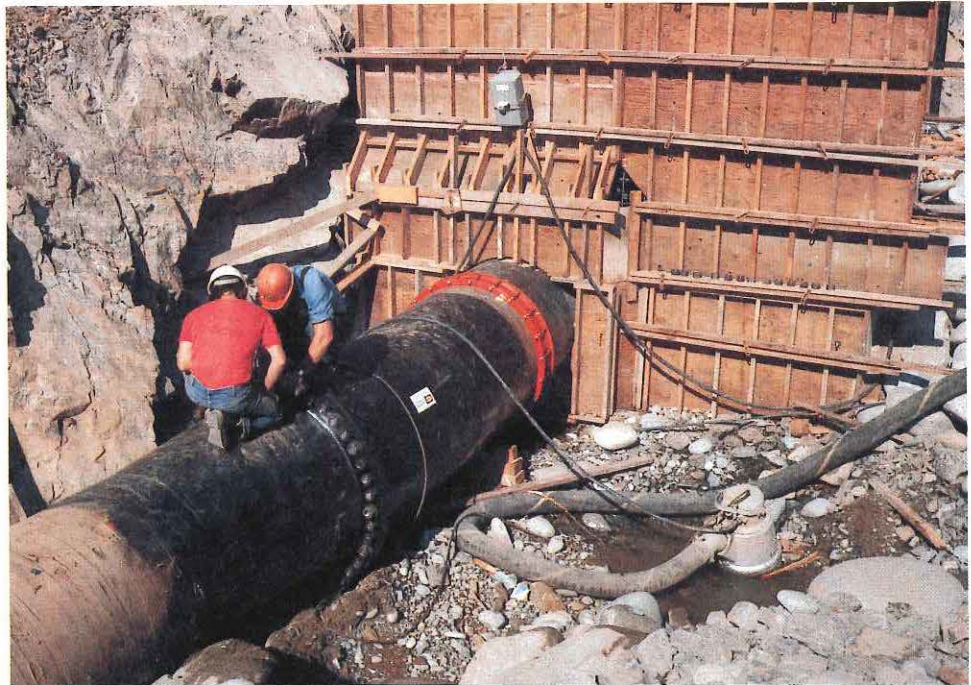
To supply the new Chehalis hatchery with water, a 106 cm pipe is installed from the concrete intake built beside the Chehalis River. (Photo: Y. Wai Leung)
