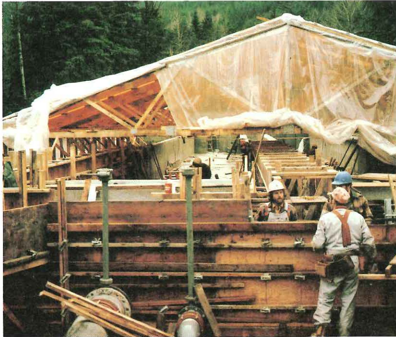
During construction of the chum rearing channels at Chilliwack, a makeshift canopy wards off December rains.
