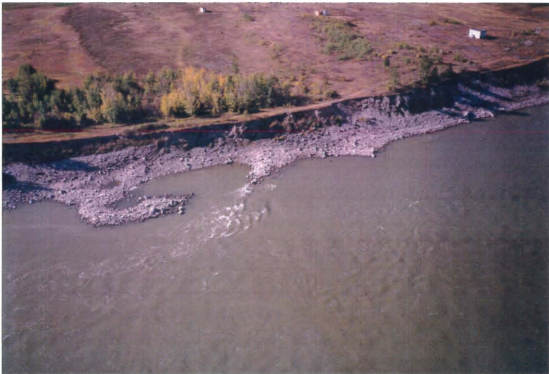
Photograph 7. Removal of riparian shrubs and trees can destabilize banks - Fraser River.
