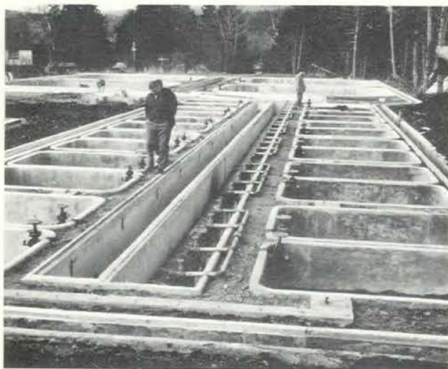
Pond arrangement built at Margaree Fish Culture Station, Cape Breton, to test a Swedish method of rearing Atlantic salmon.
