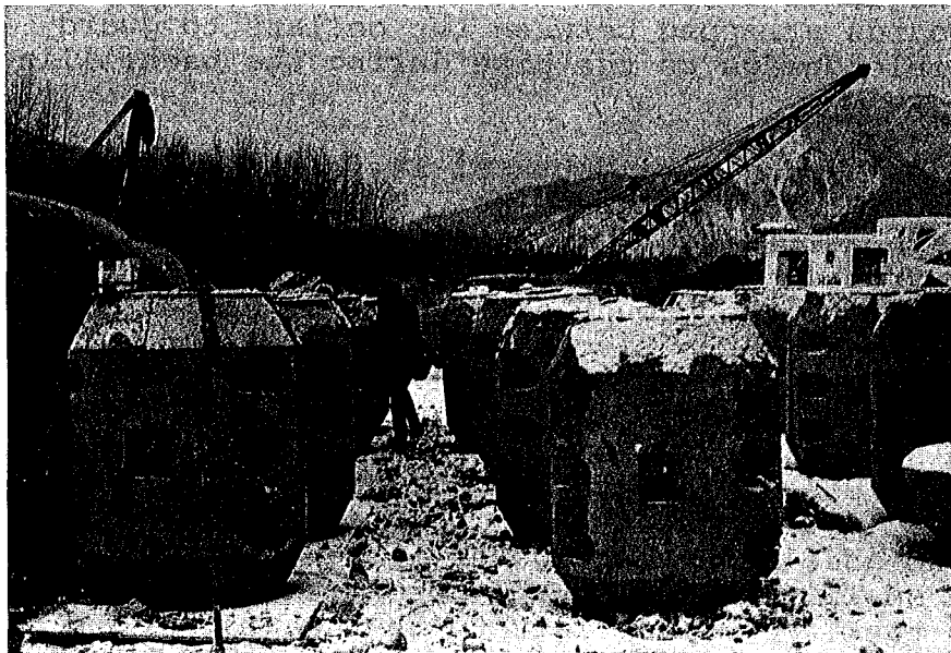
PLATE 10. Close-up of the pipeline ascending the west side of the Kotaneelee River. Note the berm and drainage breakers.
