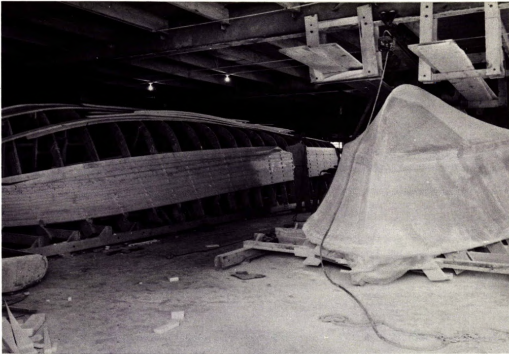
Figure 1. Core-mould system – 40-foot and 33-foot navy personnel boat hulls under construction on male forms.
